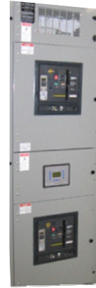
Transfer Switch without Bypass Isolation
