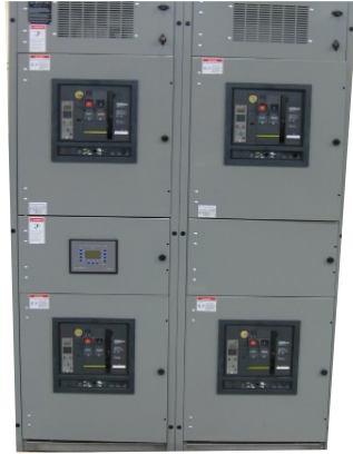
Transfer Switch with Bypass Isolation
