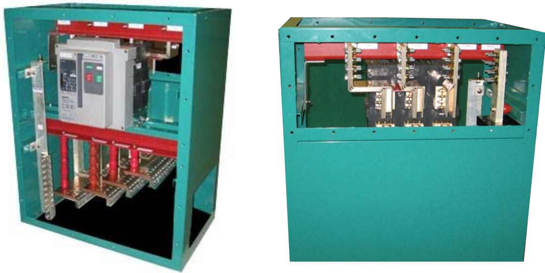
Fig. 12, Typical Single CB with Neutral Sensor, Bottom Right Hand Side Cable Connections (Front and Rear Views)
