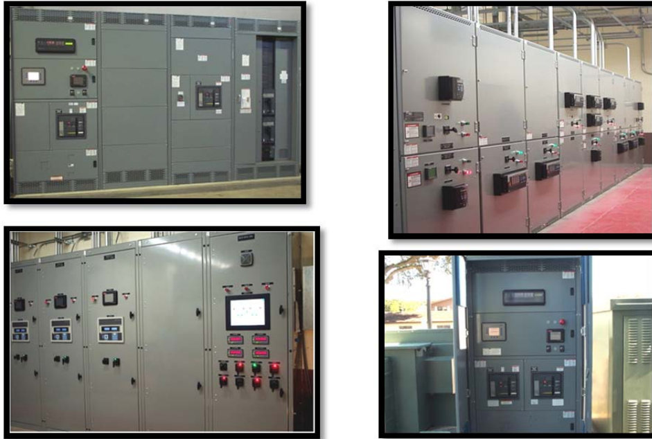
Example OSPSCS Switchgear and Control Systems
